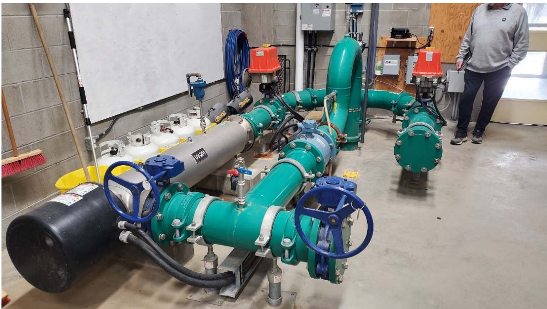
UV disinfection system for this water source at the WTP. Extra berth location for a second UV reactor is shown in the photo.
