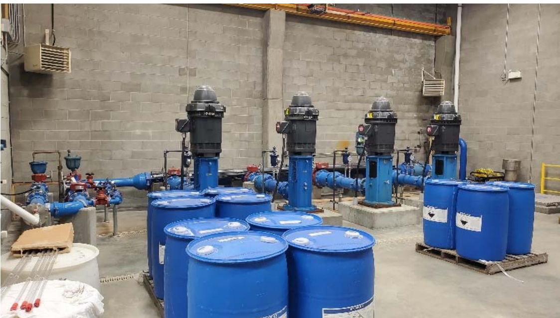
4 – 125 hp Duty Pumps that lift water from the 300m 3 clearwell up to the Million Gallon Reservoir pressure zone (PZ 327m)
