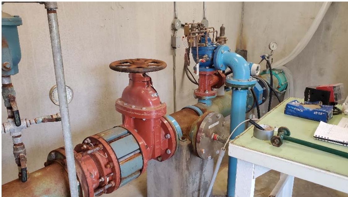
Recreation Well Building – Interior process pipe works
